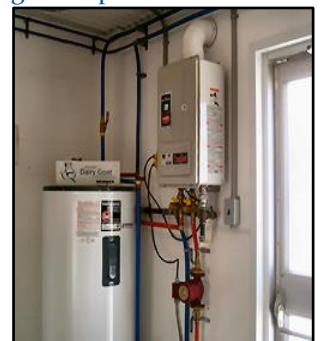
Fig. 16. Hot water tank in good repair
