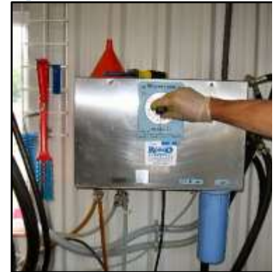
Fig. 17 Was control box in good repair
